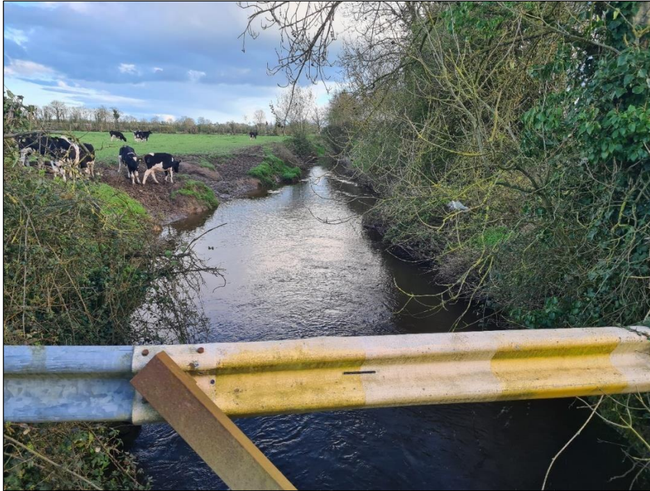
Plate 6-25 View of existing crossing at the Suir River located at the southeast of the Site leading the proposed substation location from turbine 8.
