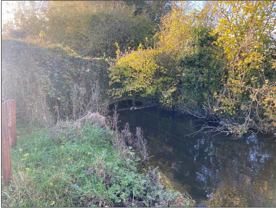
Plate 6-30 Bridge at Clonmore river where grid connection will pass underneath (HDD) within the road, southeast of the Site.
